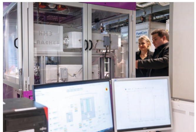
Figure 3: Demonstration plant with SOFC stack and afterburner (TOX).
